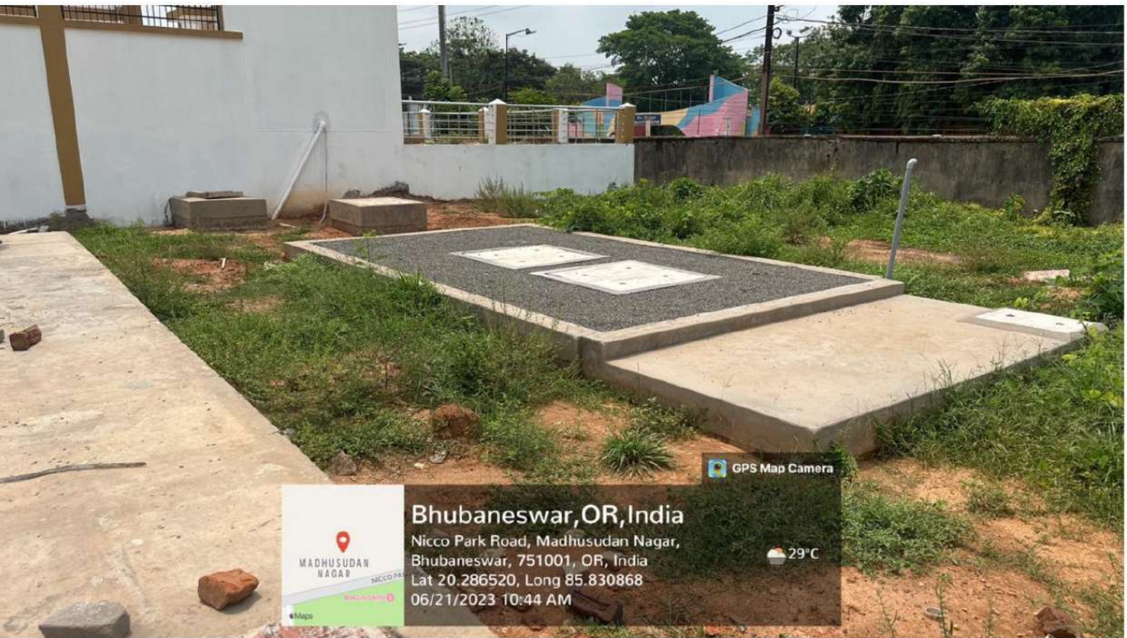
SEWAGE TREATMENT PLANT REGIONAL INSTITUTE OF EDUCATION ,BHUBANESWAR
